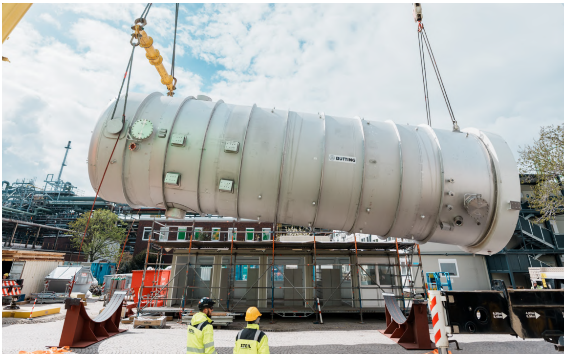
A component for one of the world's most powerful heat pumps arrives at the BASF chemical factory in Ludwigshafen, Germany.
