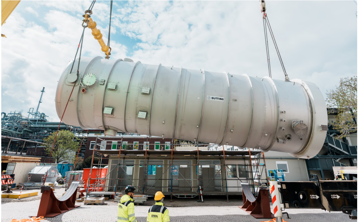
A component for one of the world's most powerful heat pumps arrives at the BASF chemical factory in Ludwigshafen, Germany.
